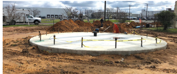
Foundation is completed and is ready for the construction of the steel water tower.
