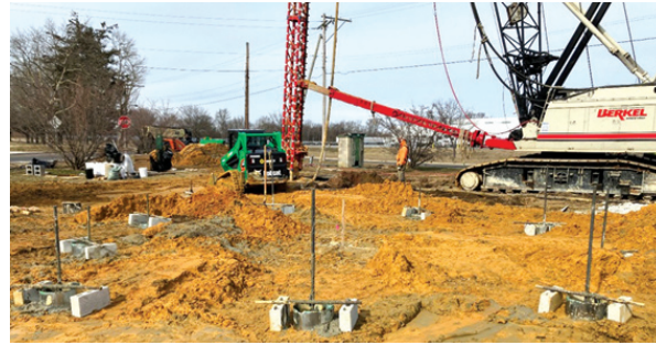
Pilings sixty to eighty feet deep have been installed for the Water Tower Foundation.
